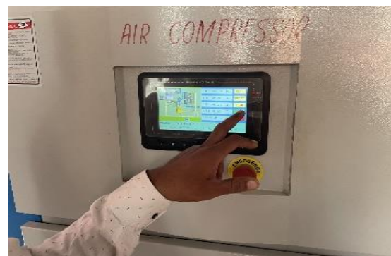
Figure 2: Technician demonstrating shut down procedure.
